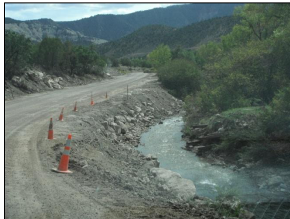
Figure 3.66 – Ongoing construction, to clean up mudflows that had crossed the Sweetwater Creek road, made the water extremely turbid in Sweetwater Creek.
