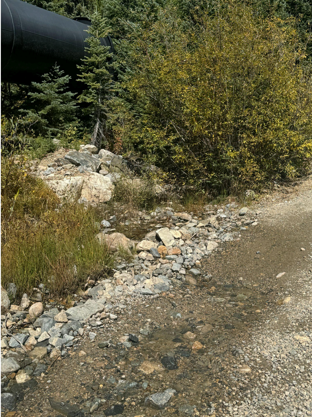
Upper Fancy Stream Crossing; Stream percolating/overbanking upstream of the culvert and spilling onto the roadway at base flow.
