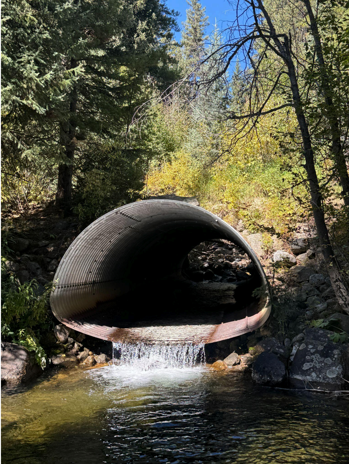
Missouri Creek Stream Crossing; Downstream Perched Outlet (39°23'52.3"N 106°26'40.2"W)
