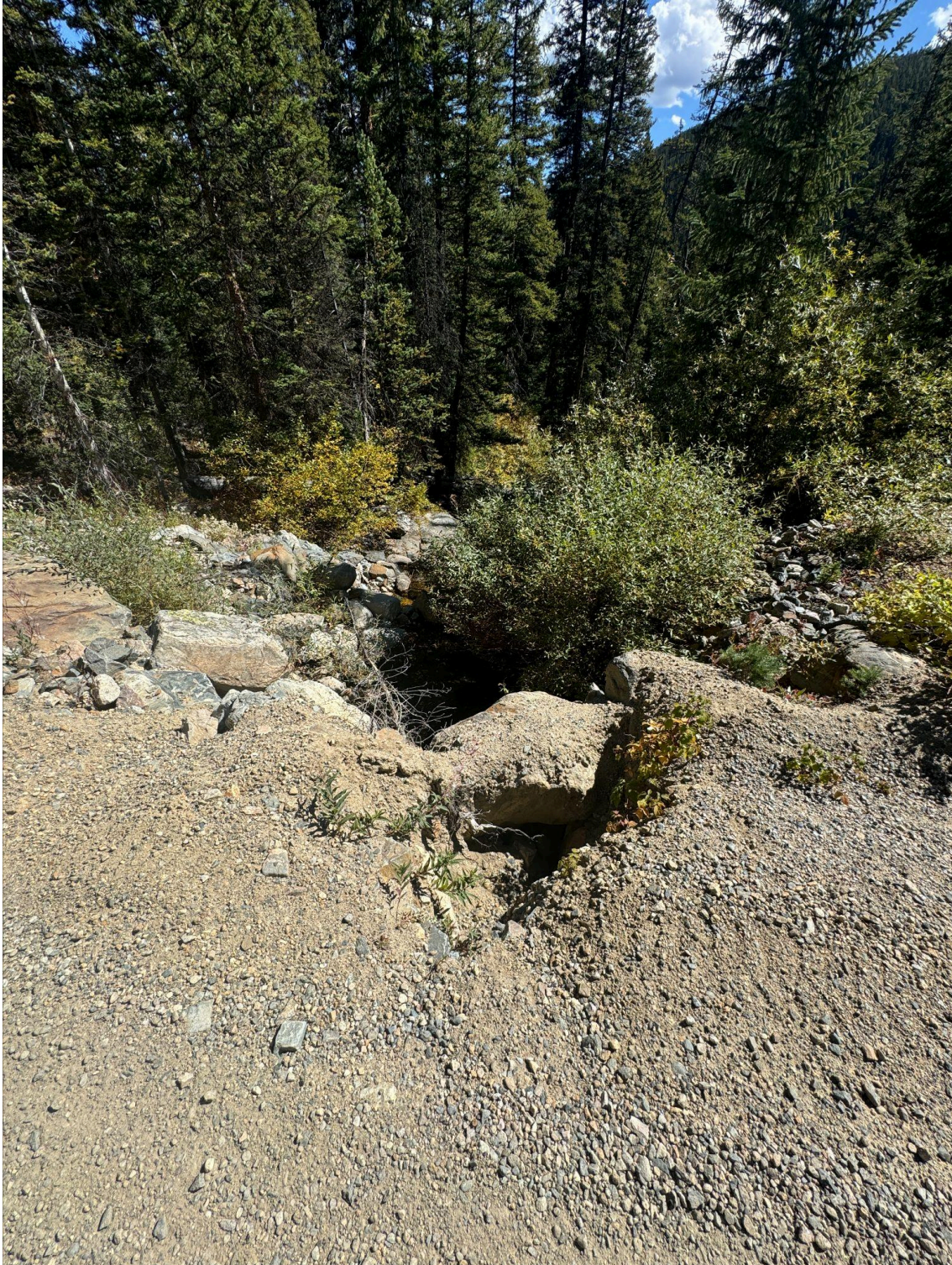
Upper Fancy Stream Crossing; Erosion/head cut at the culvert outflow. (39°23'42.7"N 106°28'12.9"W)
